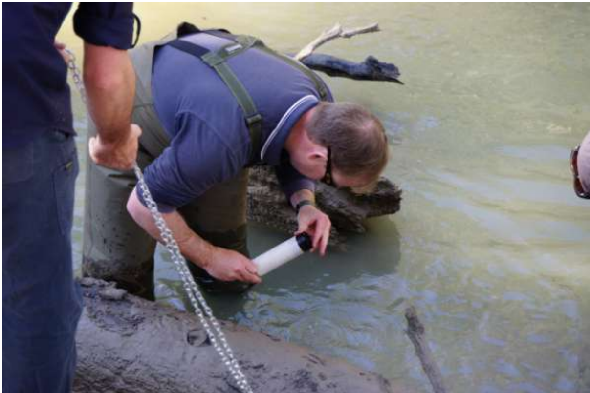
Installation of water quality monitoring equipment at Whealbah Bridge on the Lachlan River.
