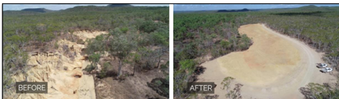
Photo: Example of a before and after photo of a degraded gully remediation to reduce erosion and sediment run-off.
