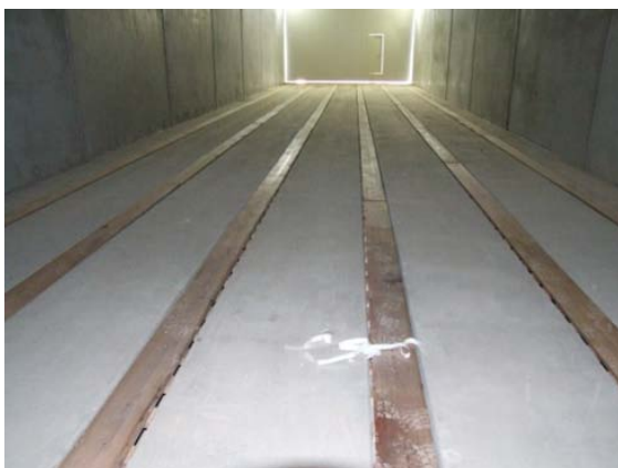
Inside a composting tunnel with aeration channels
