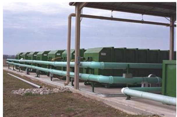
Containerised composting system
